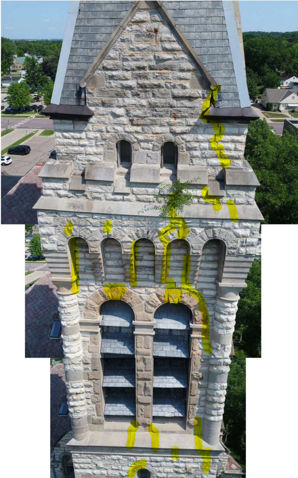
Figure 3: Cracks in South Face of the Tower.
