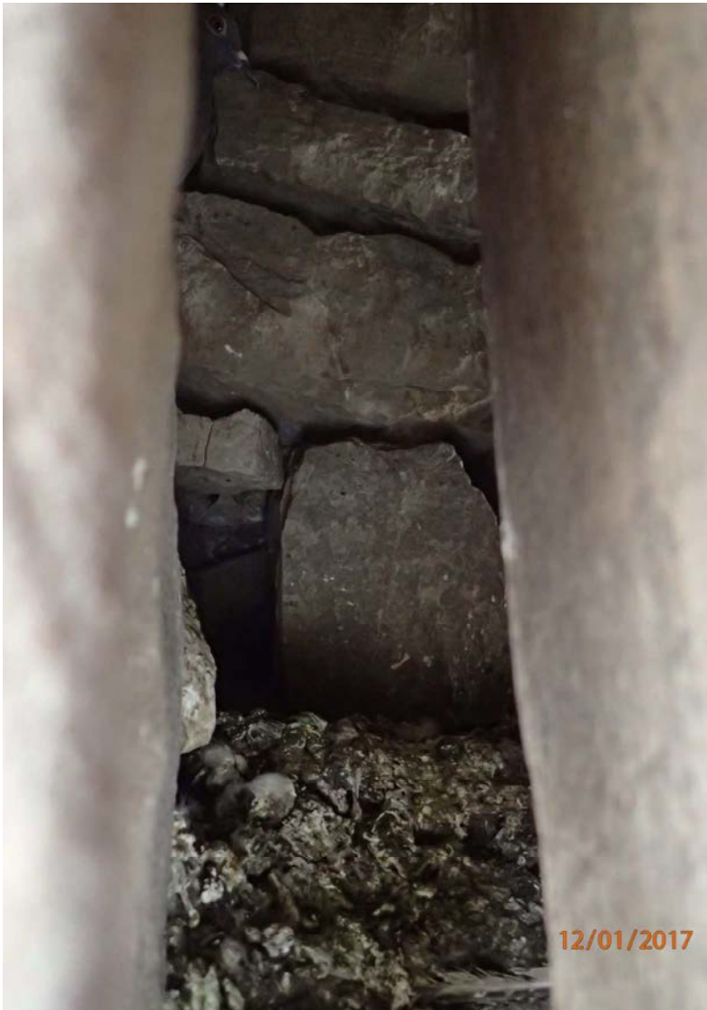
FIGURE 17: 2017 PHOTOGRAPH OF TOTAL LOSS OF ORIGINAL MORTAR IN SW CORNER OF TOWER.
