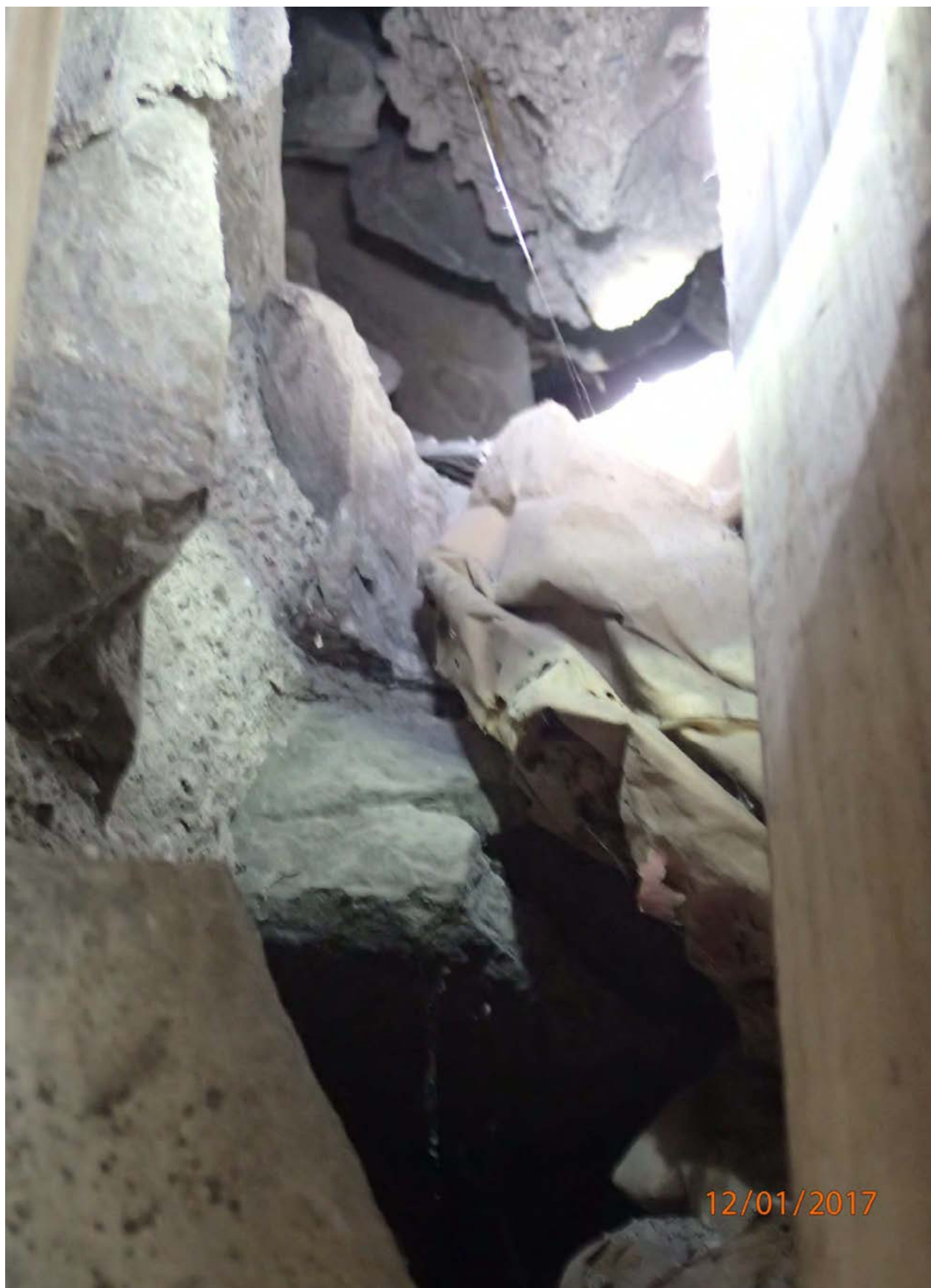
FIGURE 19: 2017 PHOTOGRAPH OF MORTAR LOSS AND WALL COLLAPSE AT CORNER OF TOWER.
