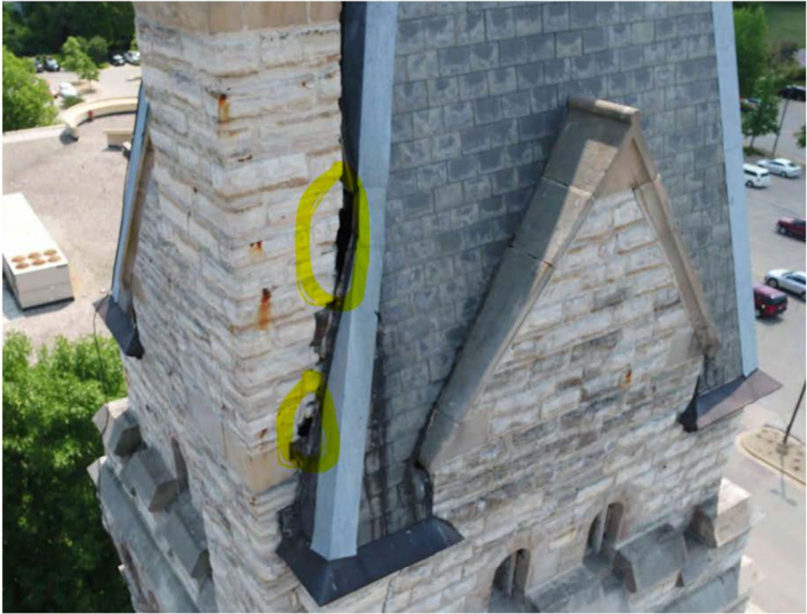
Figure 20: Gaps at Chimney Flashing.
