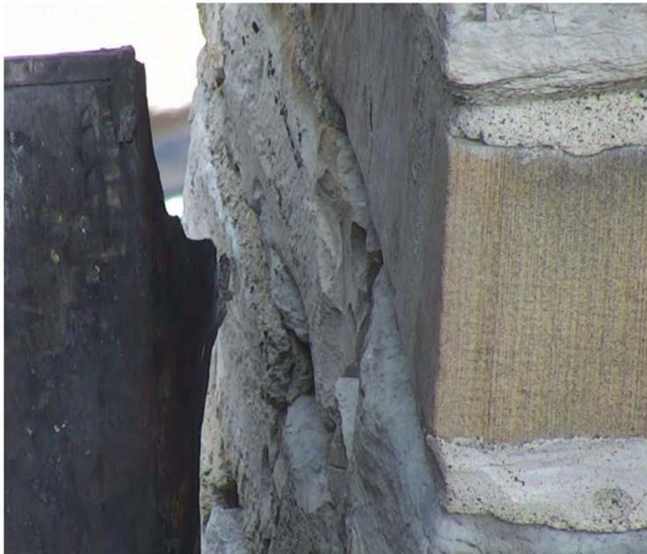
Figure 21. Mortar loss at back of Chimney.
