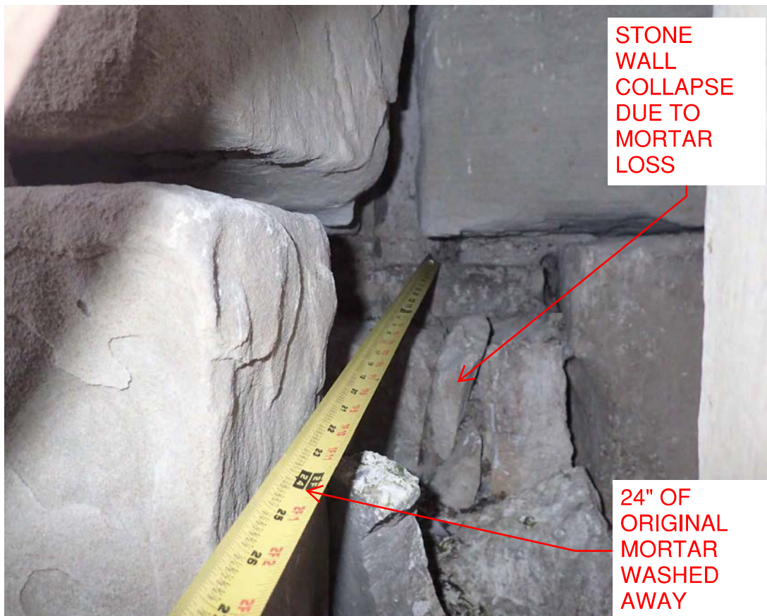
FIGURE 16: 2017 MORTAR LOSS AT NORTH EAST CORNER OF TOWER
