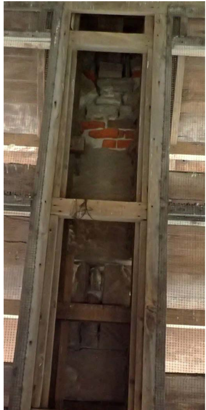
FIGURE 18: 2017 PHOTOGRAPH OF DETERIORATION IN VERTICAL SUPPORT BETWEEN LOUVERED WINDOWS IN EAST FACE OF TOWER.
