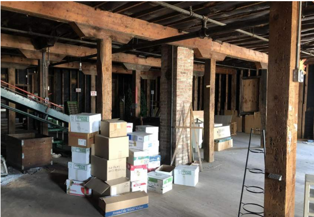
FIGURE 4 - TYPICAL WOOD FRAMING SEEN THROUGHOUT MOST OF THE BUILDING. A MAJORITY OF THE FRAMING IS IN GOOD CONDITION EXCEPT WHERE ROOF LEAKS ARE CAUSING MOISTURE INTRUSION AND DAMAGE.
