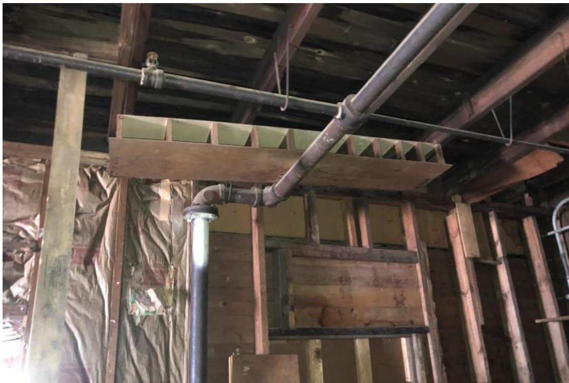
FIGURE 2 - DAMAGED ROOF FRAMING ABOVE 3RD FLOOR. PIPE IS SUPPORTING THE ROOF JOIST. ROOF IS LEAKING AT THIS LOCATION.
