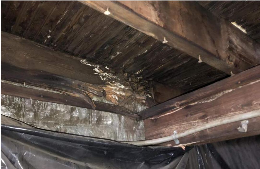
FIGURE 3 - DAMAGED FRAMING DUE TO LEAK IN ROOF ABOVE FOURTH FLOOR IN EAST WING. REPAIRS ARE NEEDED AS SOON AS PRACTICAL..
