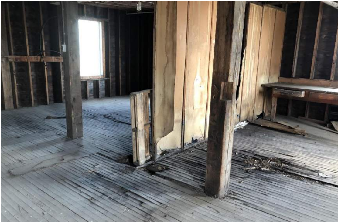
FIGURE 1 - DAMAGED FLOOR BOARDS AND JOISTS RESULTING FROM LEAKS ON ROOF ABOVE 6TH FLOOR.
