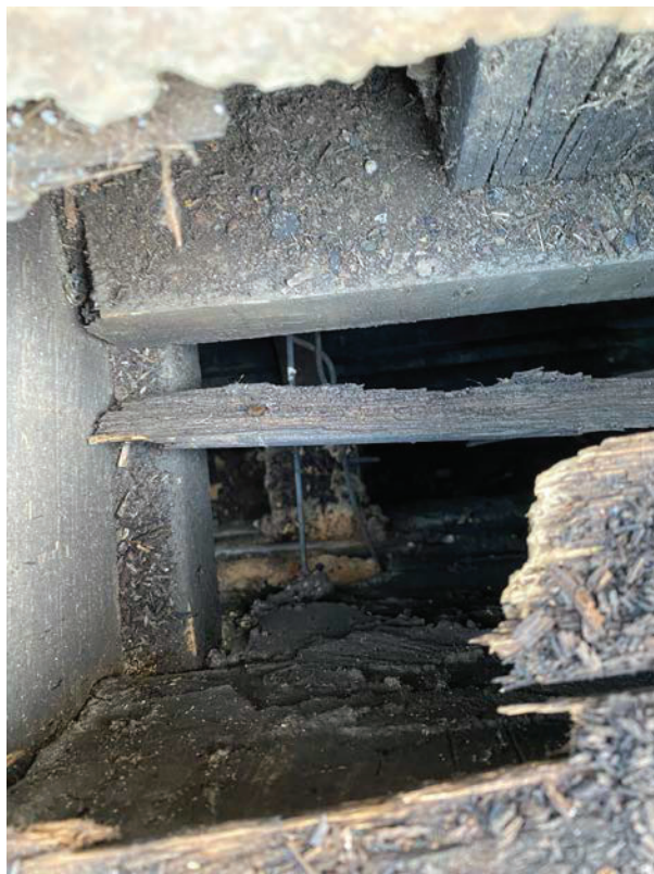
Picture 4: Existing rotted parapet and overhang framing.
