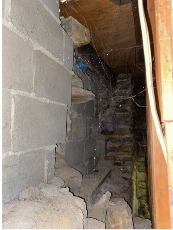
Picture 1: Existing infill in foundation wall with voids.
