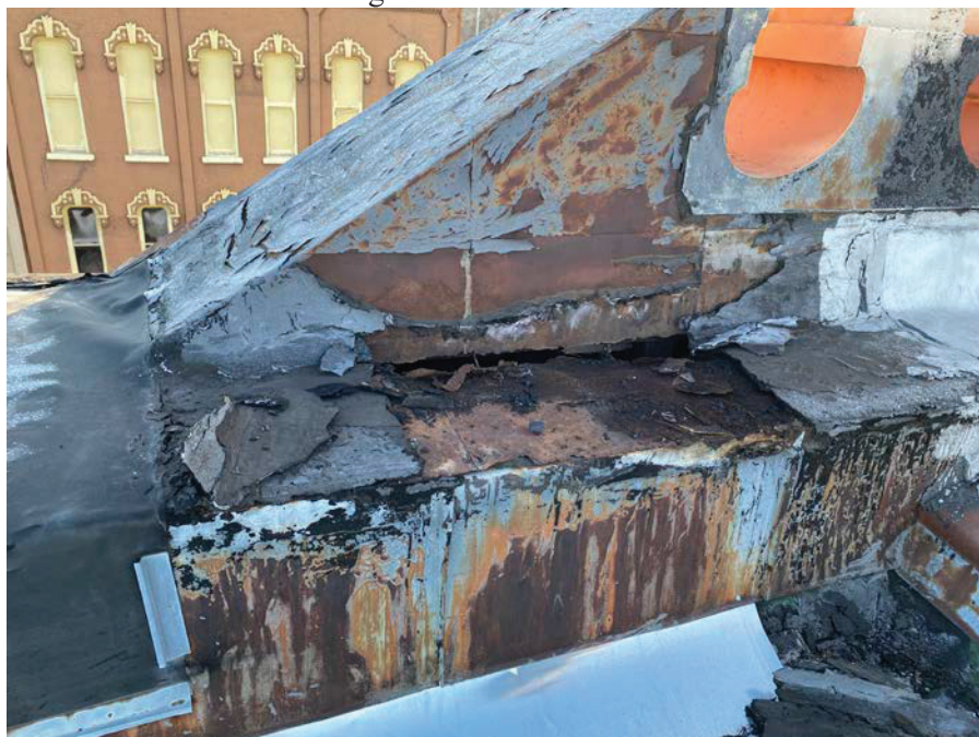
Picture 2: Existing rusted decorative parapet and overhang.
