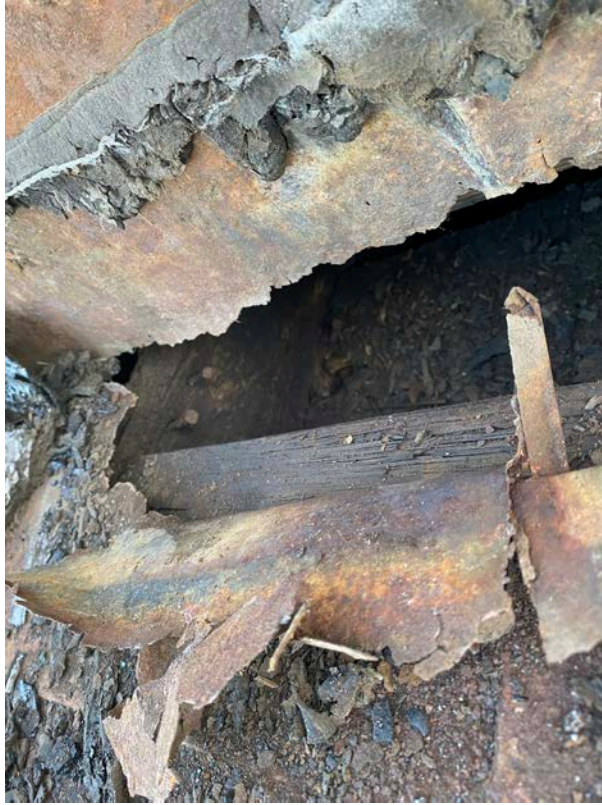
Picture 3: Existing rotted parapet and overhang framing.
