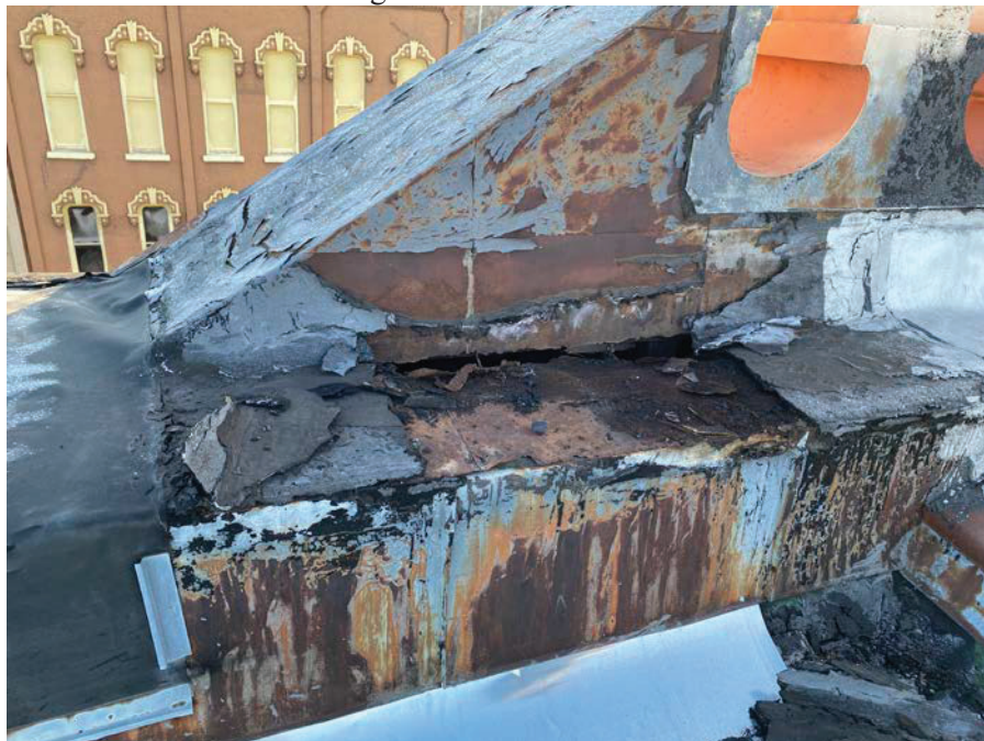
Picture 2: Existing rusted decorative parapet and overhang.
