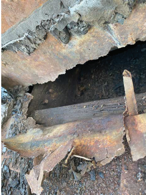
Picture 3: Existing rotted parapet and overhang framing.
