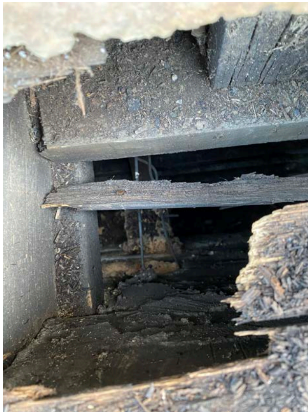
Picture 4: Existing rotted parapet and overhang framing.
