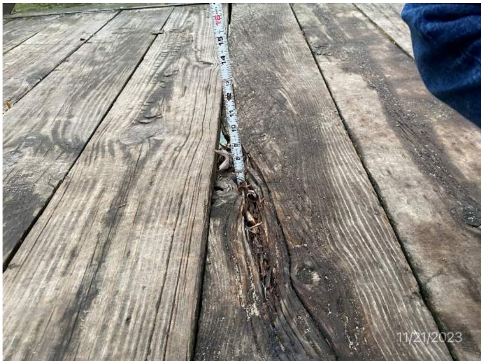
Damaged timber plank, 18 th from the south
