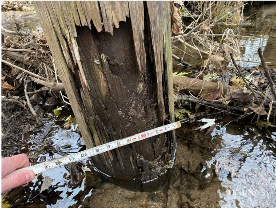
Moderate decay and section loss at pile 2, Pier 3, looking east
