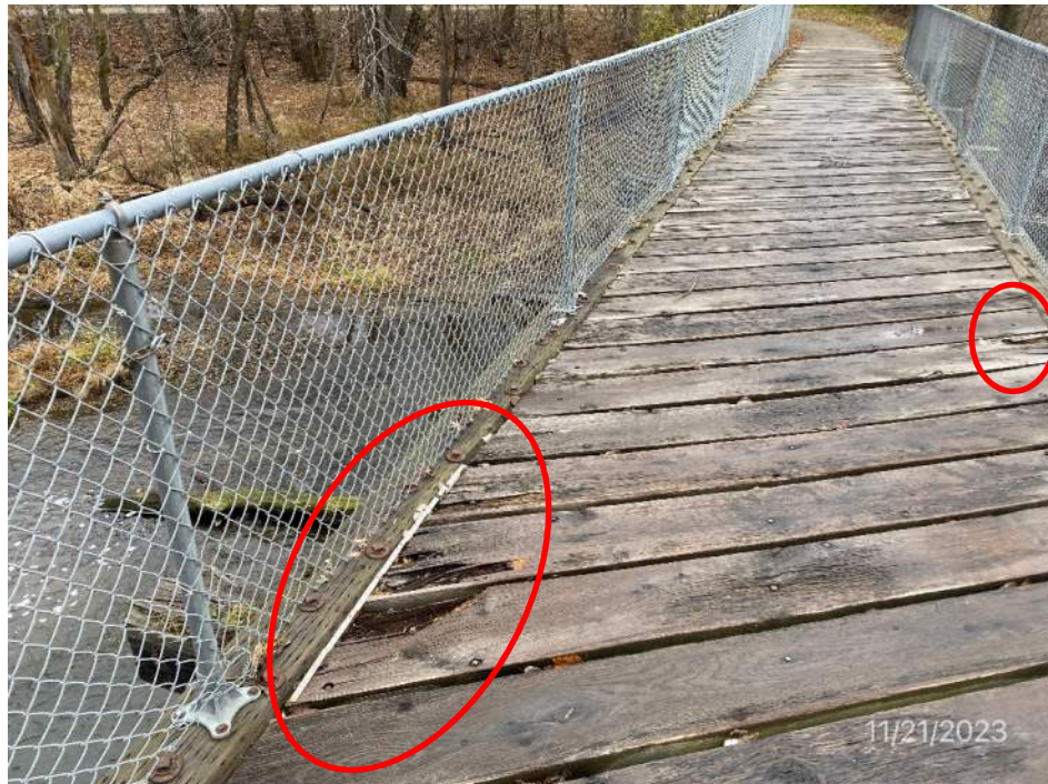
Decay and section loss in timber deck planks near midspan, looking south
