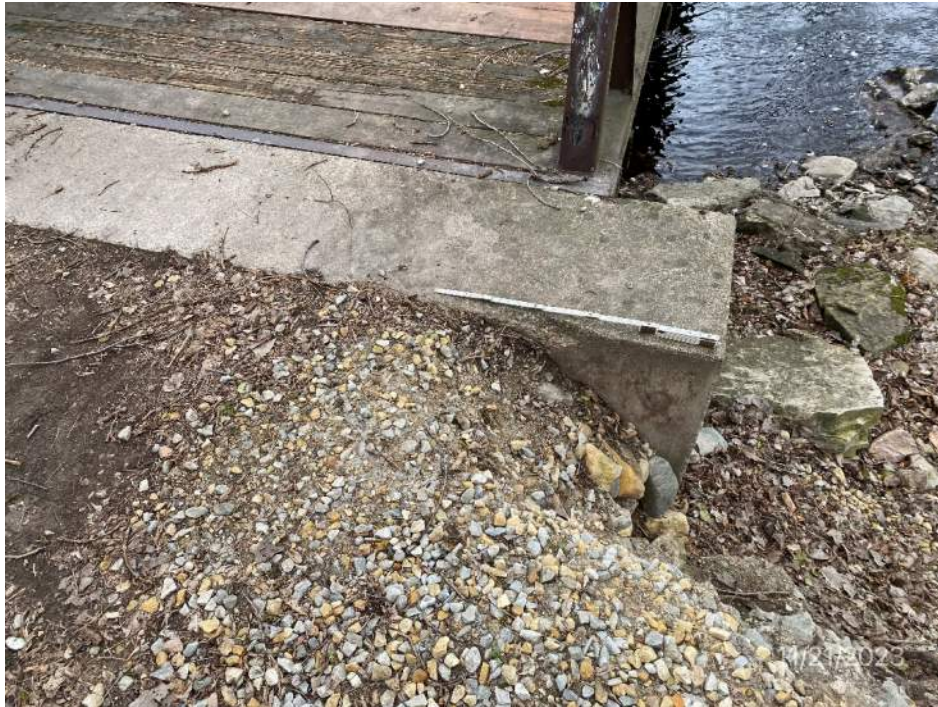
Erosion at southeast abutment corner
