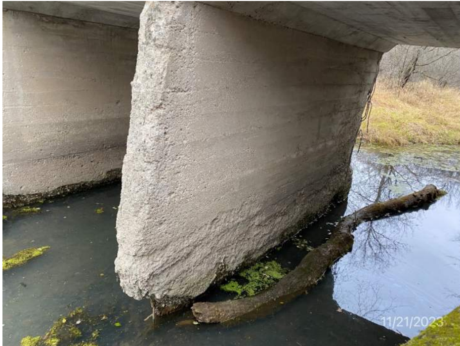
Damaged center wall with large spalls and exposed reinforcement, looking northeast
