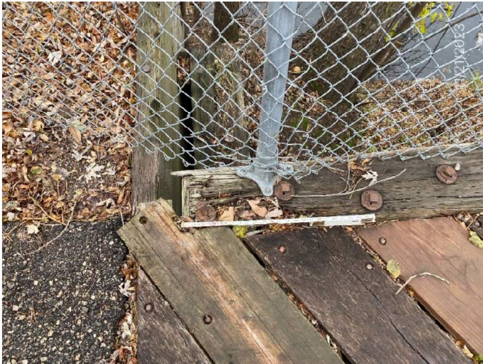
Damaged timber curb and loose rail post connection at southwest corner
