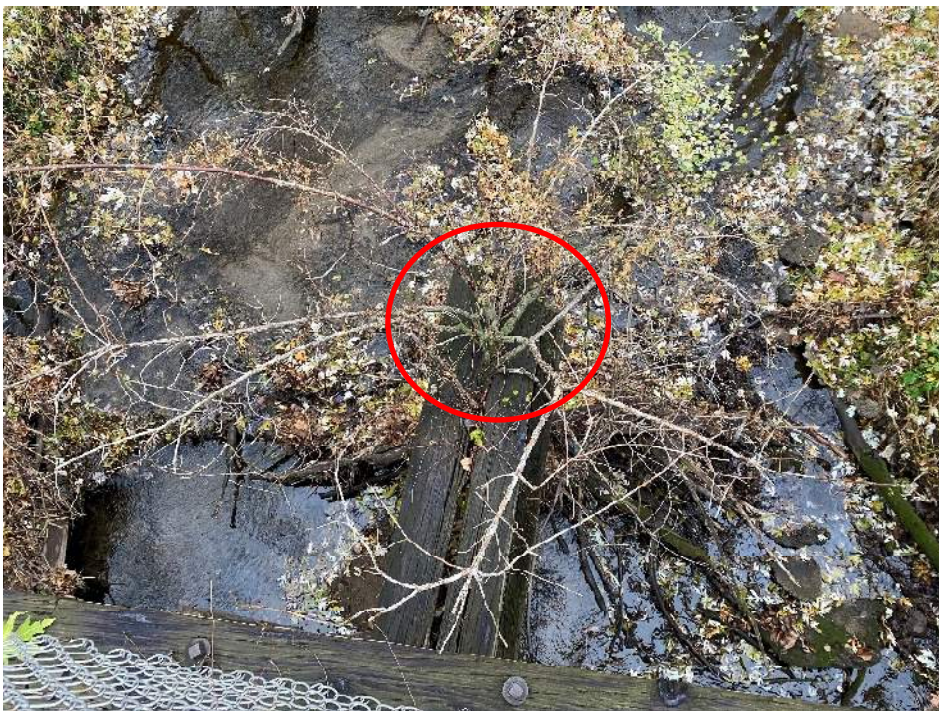
Plant growing from top of Pier 3 timber pier cap, north side, looking down
