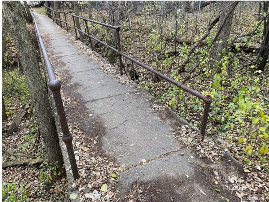
Bridge deck with missing rail section at northeast corner of bridge, looking northwest
