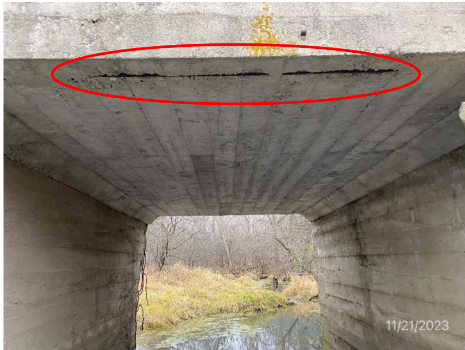
Spall with exposed reinforcement in south cell looking east
