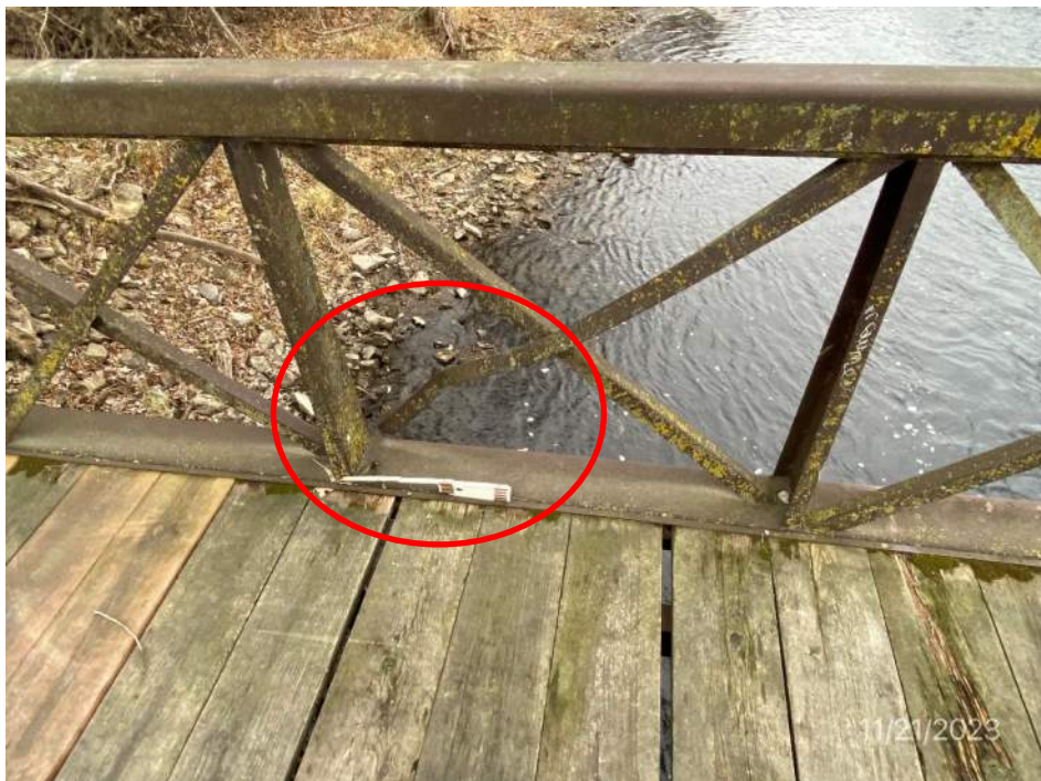
Broken rail diagonal along west rail, 5 th bay from the south
