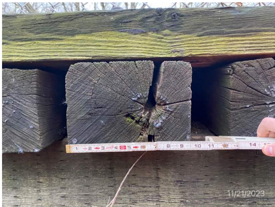
Typical end checks and splitting of timber floor beams
