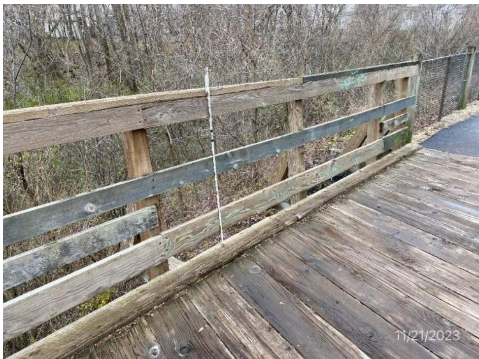
Missing rail planks at southeast corner of the bridge
