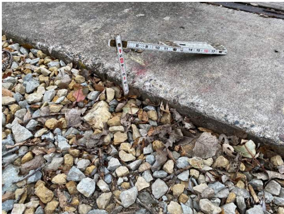
Settlement of trail at north abutment
