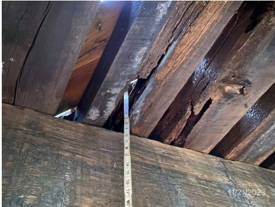
Severe decay and section loss to two floor beams at Span 3, Pier 2
