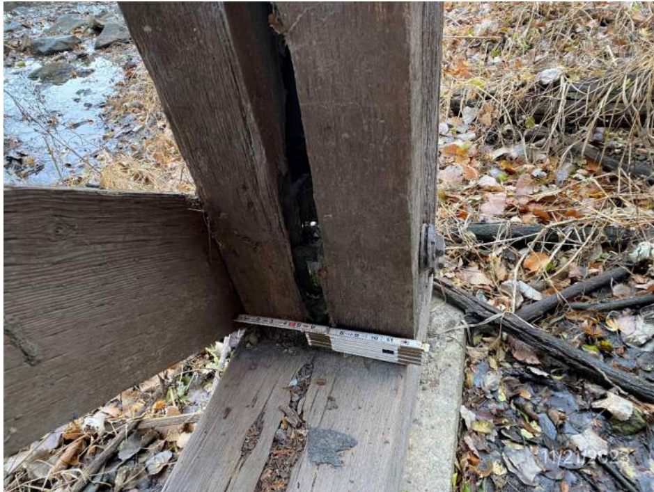
Severe decay and section loss at west timber column at Pier 4, looking west
