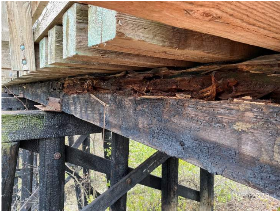
Severe decay and section loss along Beam 6 in Span 7, looking south
