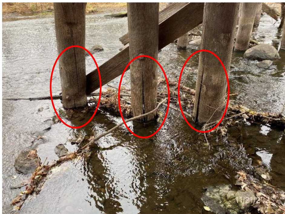
Severe decay and section loss to bottom of timber columns 4, 5, and 6 from west at Pier 6
