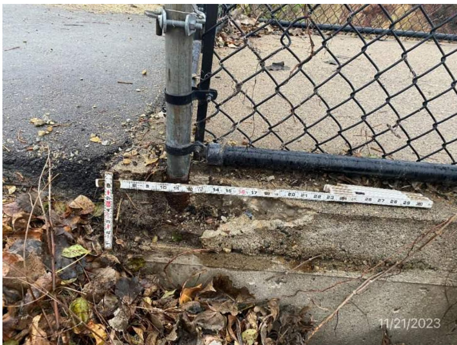
Spall with exposed rail end post anchorage at northeast corner
