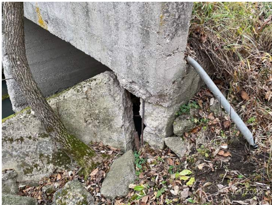
Broken wingwall at southwest corner
