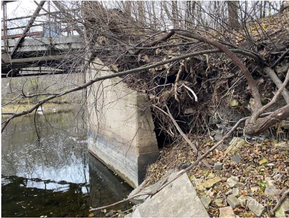
Erosion behind northeast wingwall
