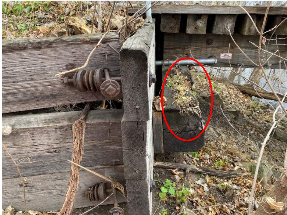
Decay and section loss to top of north abutment pile cap, looking east
