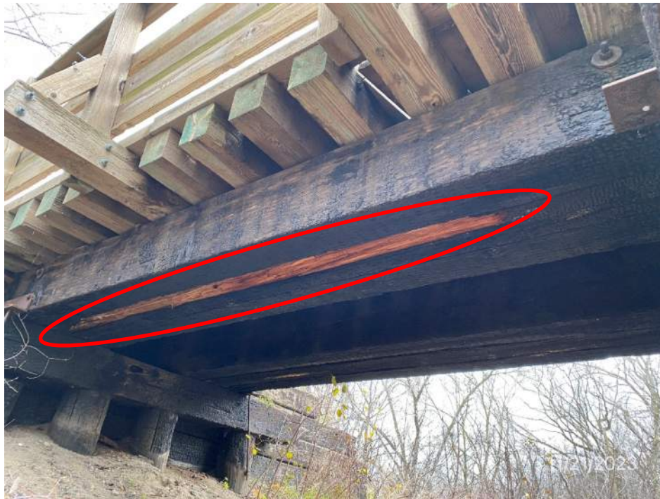
Decay and section loss to bottom of Beam 2 in Span 7, looking east
