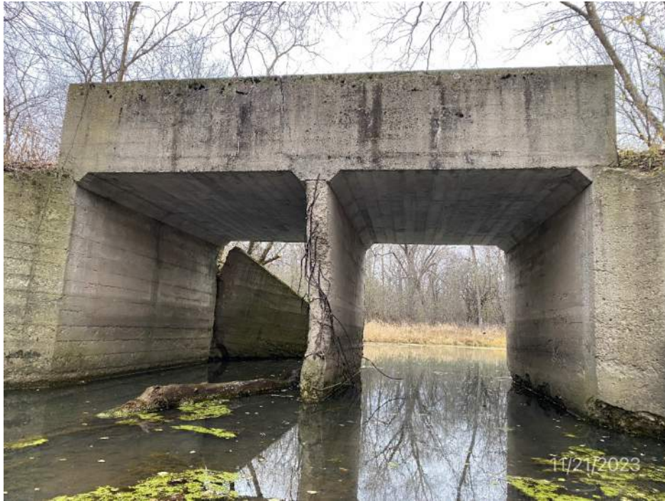
Large spall with exposed reinforcement at east side of center wall, looking west
