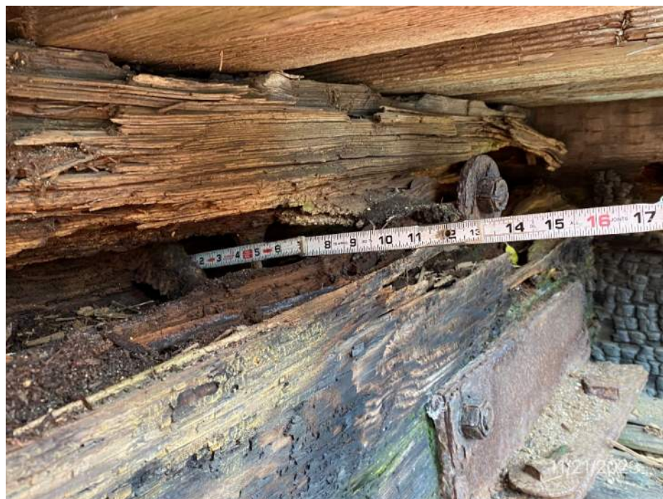
Severe decay and section loss to Beam 6 at North Abutment, looking north
