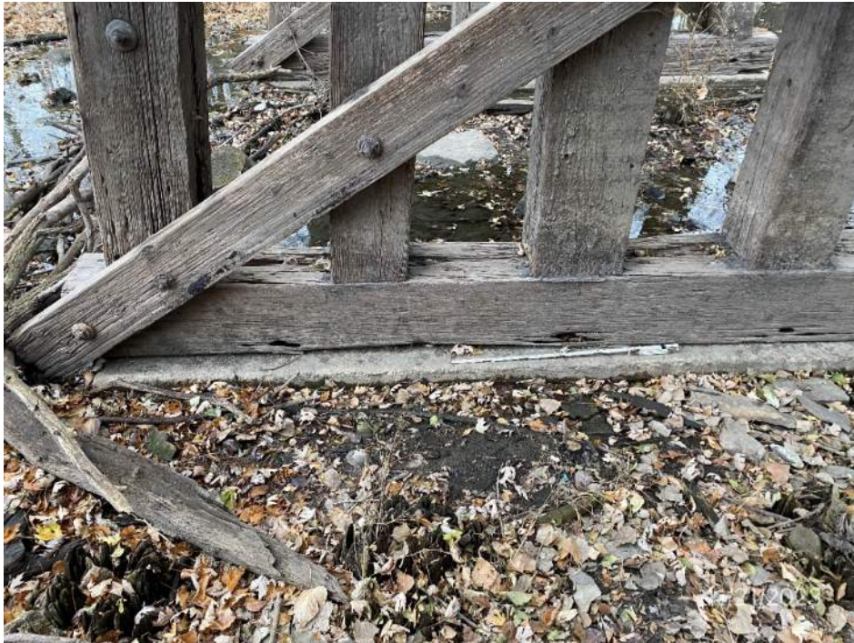
Severe decay and section loss at base of timber columns and timber footing at Pier 2, looking north
