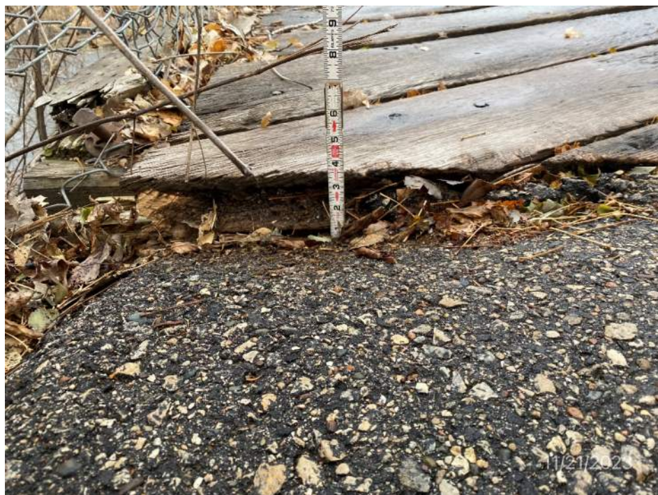
Settlement of approach pavement at northeast corner
