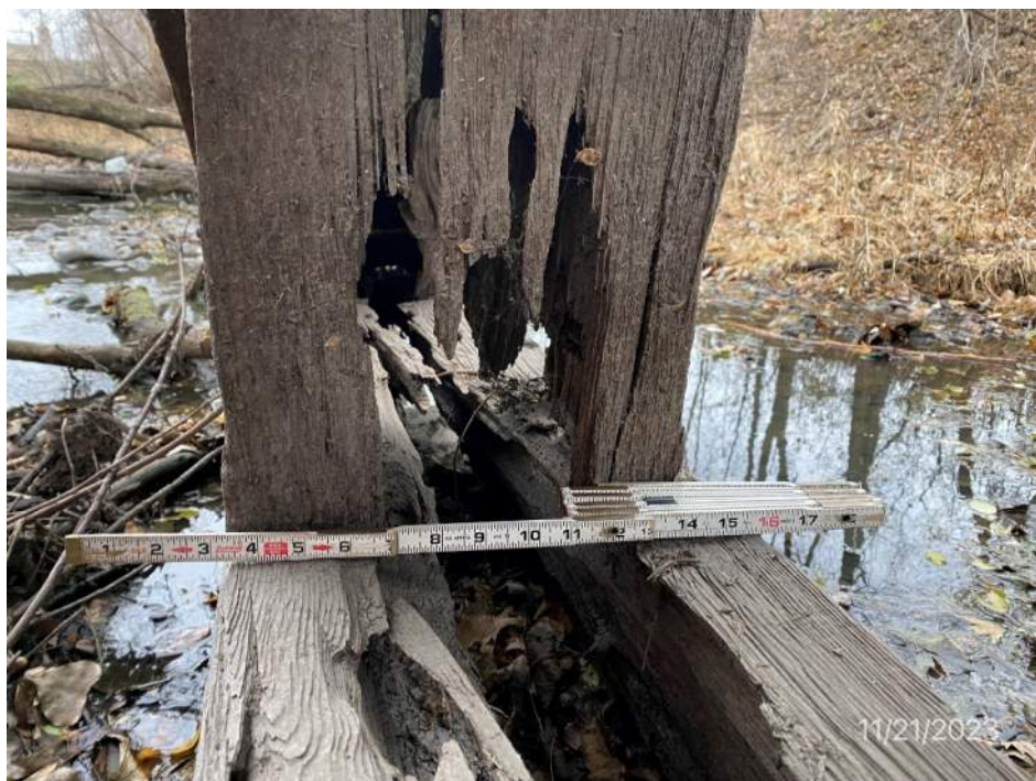
Severe decay and section loss to bottom of 2 nd timber column from west at Pier 3
