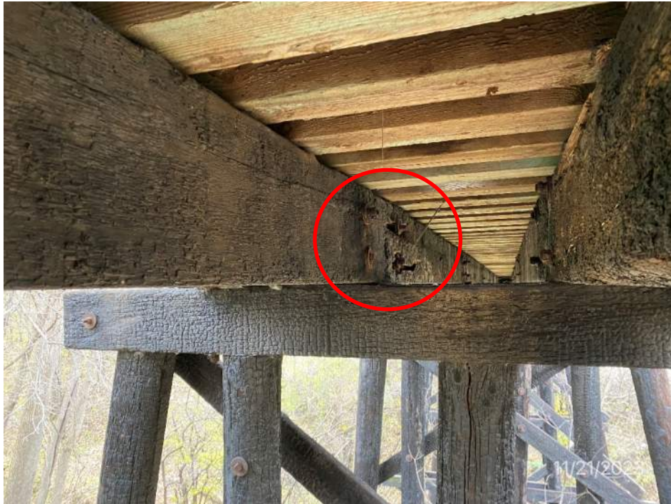
Span 1 looking north. Severe decay and section loss to Beam 3 at Pier 1
