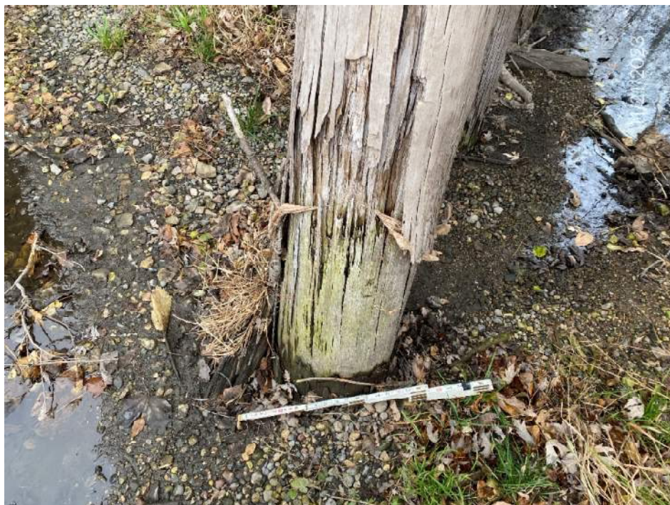
Decay and section loss at Pier 2, west timber pile
