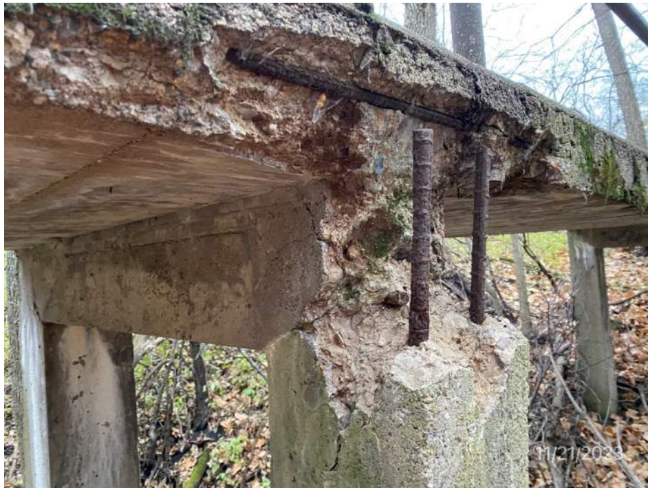
Damaged north column and slab at Pier 2, looking southwest
