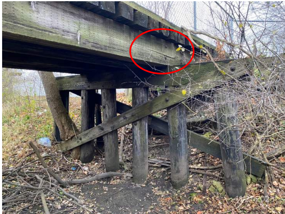
Horizontal split in Beam 8 at Pier 1, looking west
