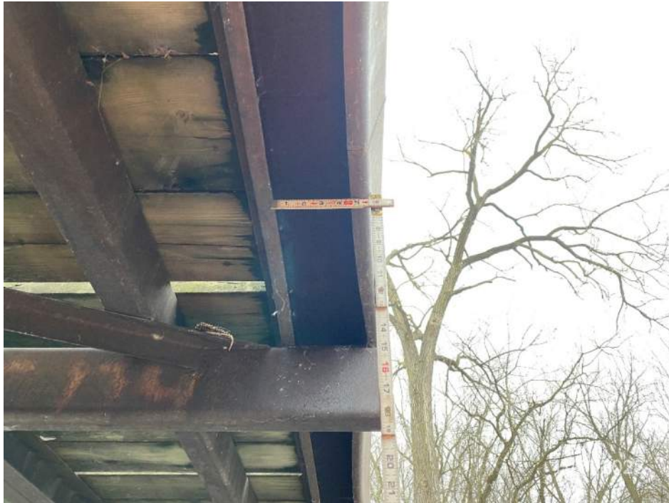
Minor impact damage to west exterior channel, looking south
