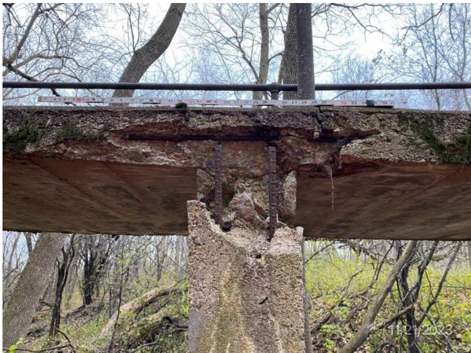
Damaged north column and slab at Pier 2, looking south
