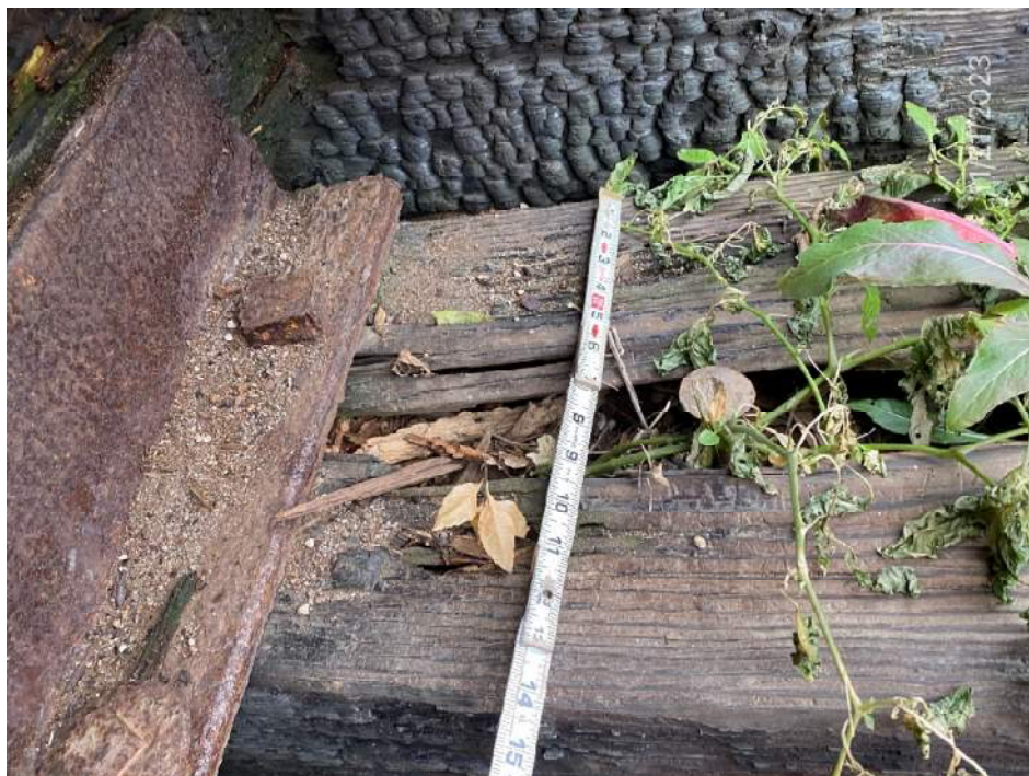
Decay and section loss to North Abutment pile cap at east end
