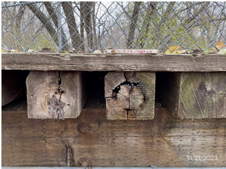
Typical end checks, splits, and decay to timber floor beams
