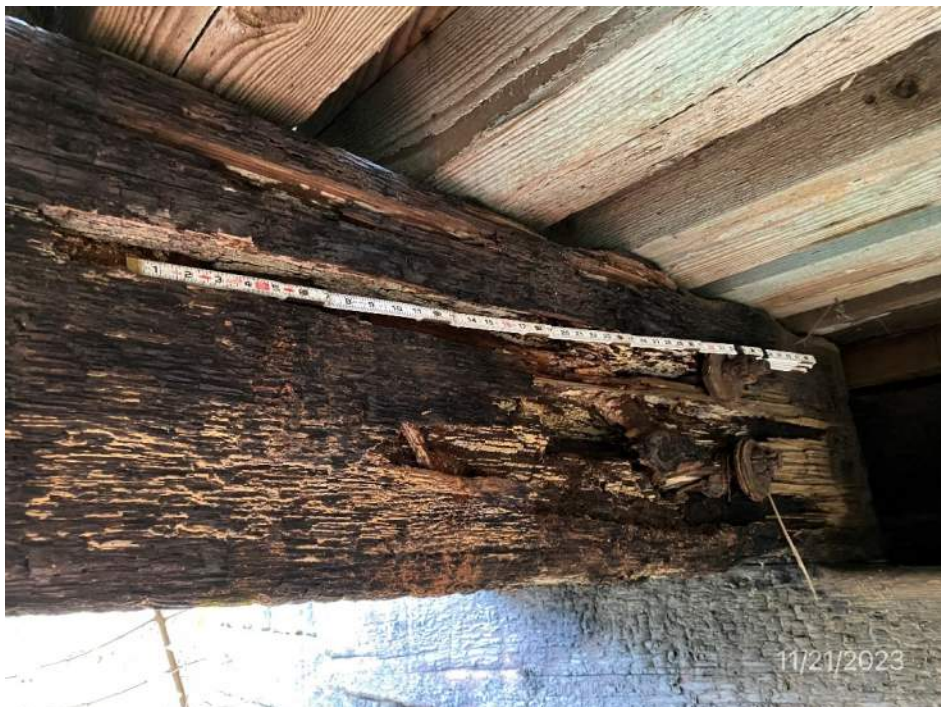
Severe decay and section loss to Beam 4 near South Abutment.
