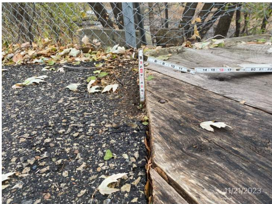
Settlement of approach pavement at north approach
