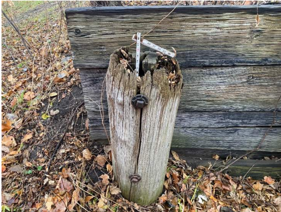
Severe decay and section loss at southeast wingwall pile, typical at all wingwall piles
