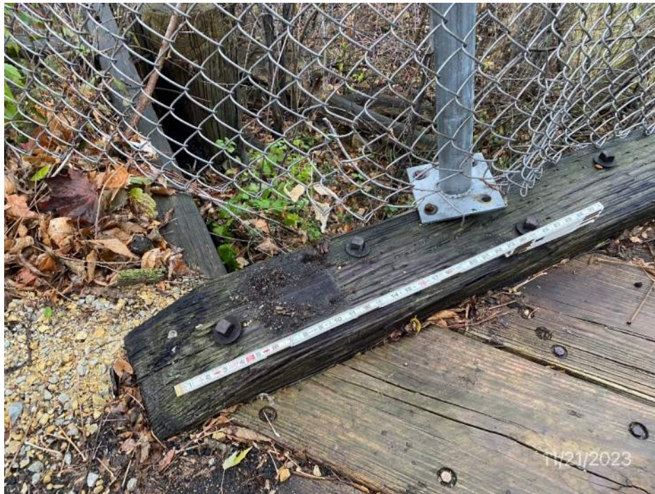
Rail end post at northwest corner with failed connection
