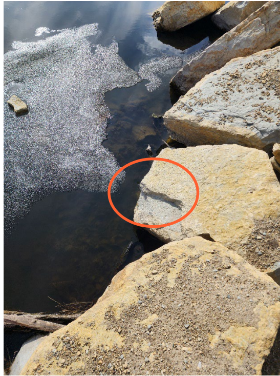
Photograph 8 Vortex Upstream of the Left Abutment
