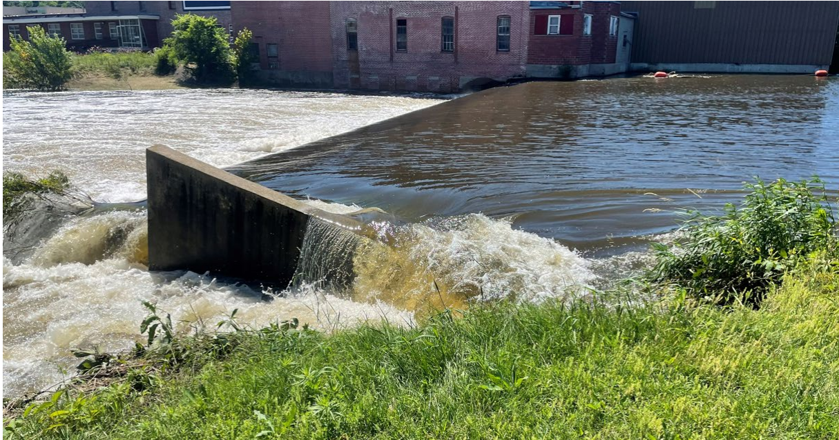
Photograph 4 Water Flowing Over Top and Around the Wall
