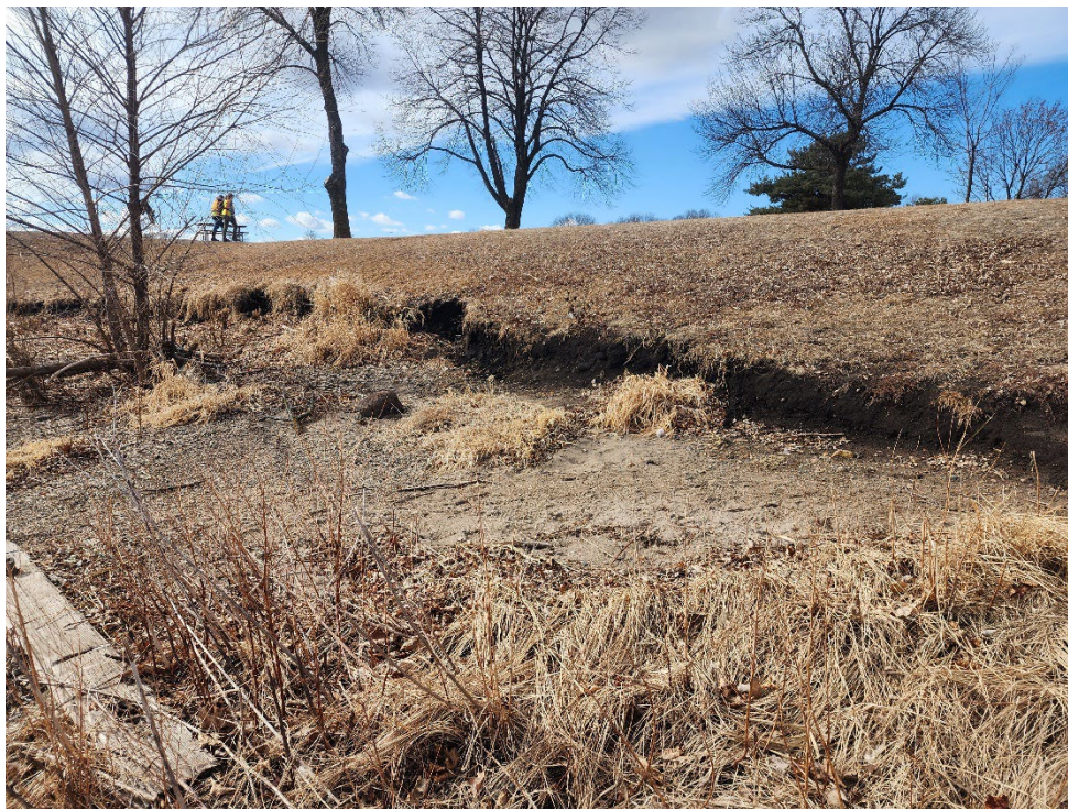
Photograph 4 Erosion on the left Embankment of the South Dam
