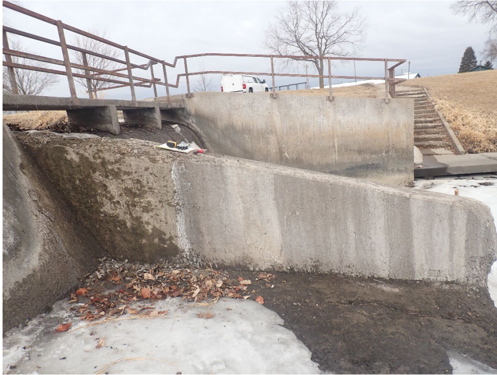
Photograph 26 Delaminated Concrete On Left of Concrete Dividing Wall and Spalled Concrete on Right (Facing North)
