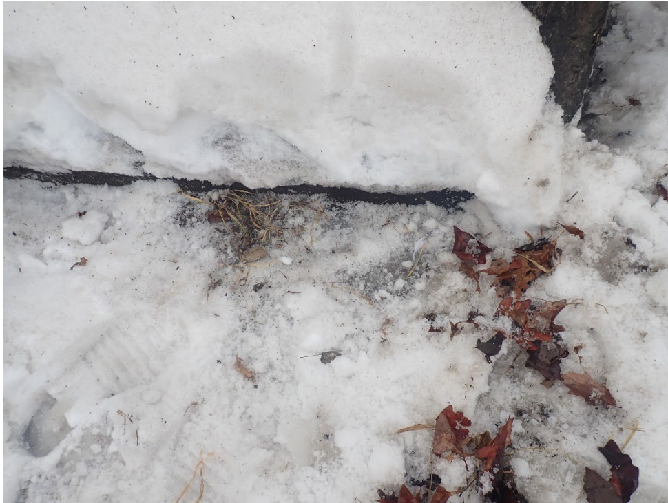
Photograph 20 Vegetation Growth in Joint Between the Downstream Edge of Concrete Dam and the Base Slab
