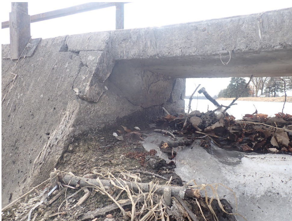
Photograph 23 Example of Spalled Concrete Near Access Slab Connection to Gravity Dam
