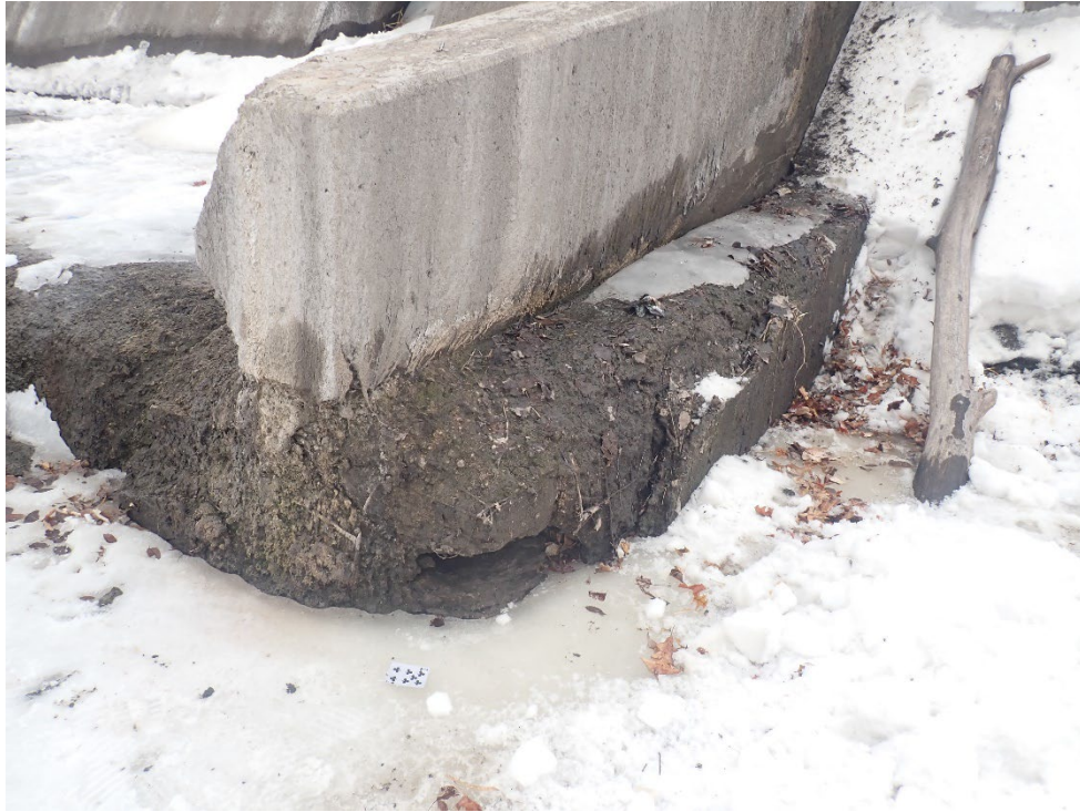
Photograph 24 Spalled and Delaminated Concrete Between Right Stop Log Section and Left Overflow Section
