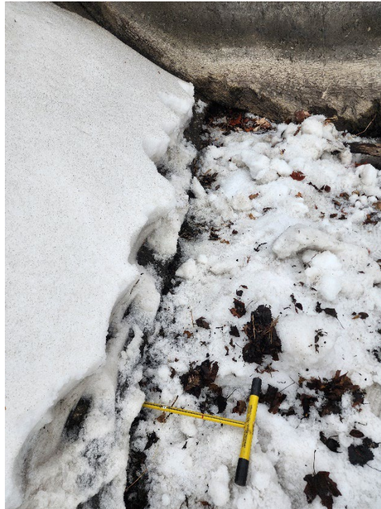
Photograph 21 Undermining in Joint Between the Downstream Edge of Concrete Overflow Section and The Base Slab
