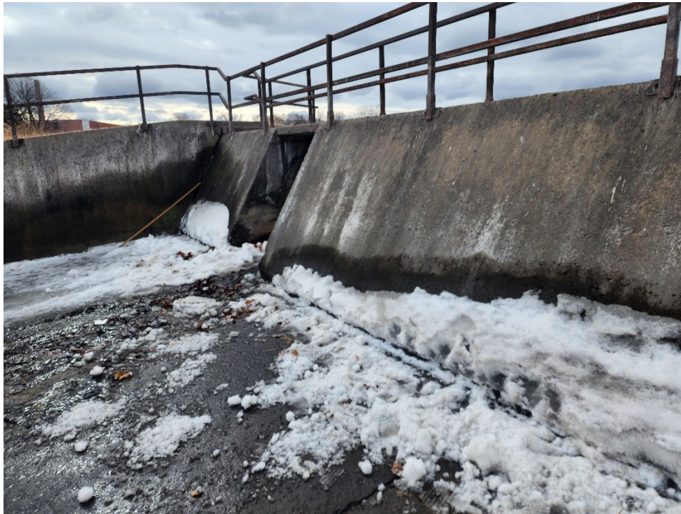
Photograph 19 Typical Joint Between the Downstream Edge of Concrete Dams and the Base Slab
