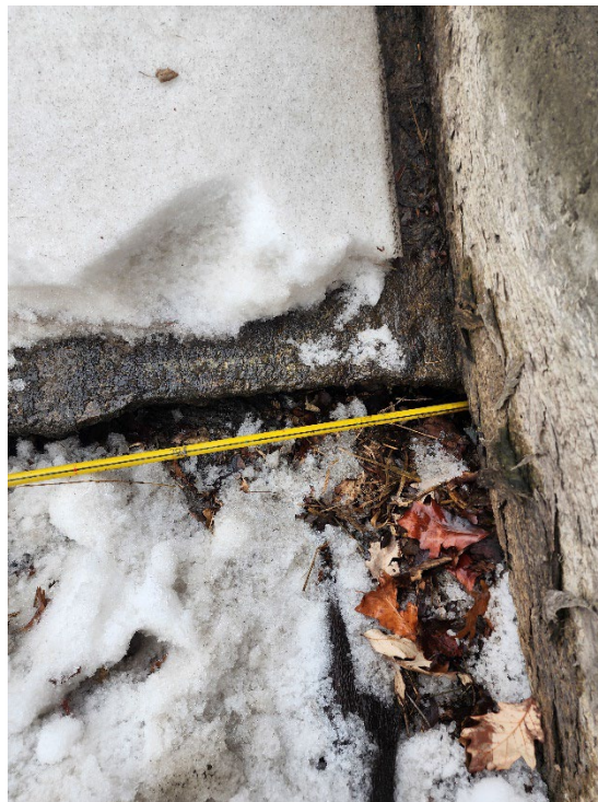
Photograph 22 Undermining in Joint Between the Left Wingwall of Concrete Overflow Section and the Base Slab
