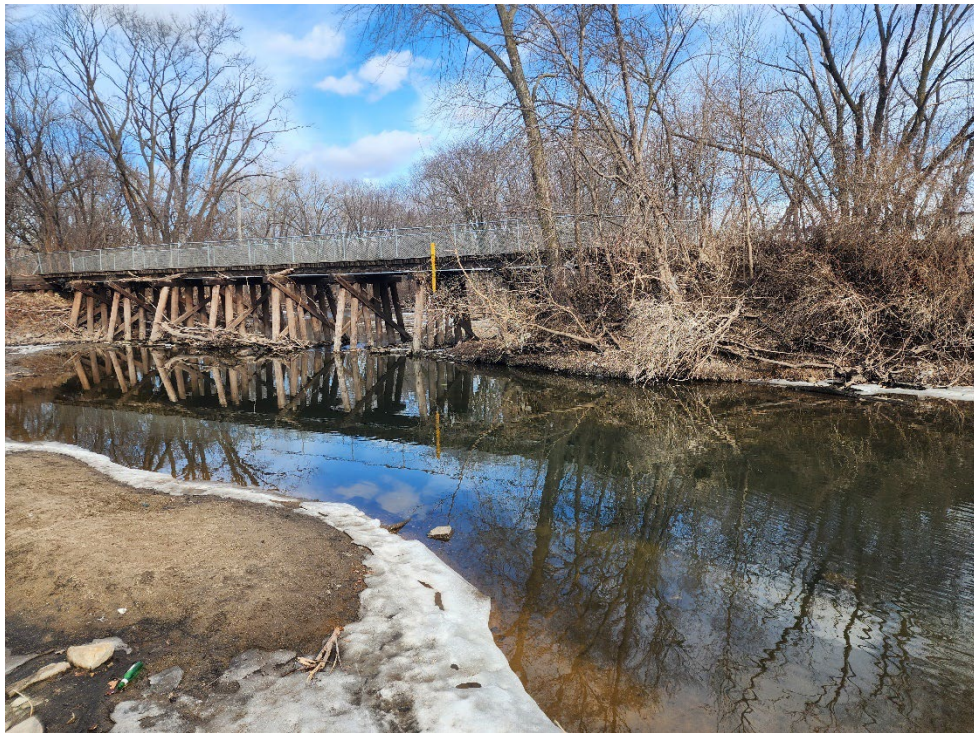
Photograph 6 Timber Bridge Downstream from the 2nd Ave Bridge and the South Dam
