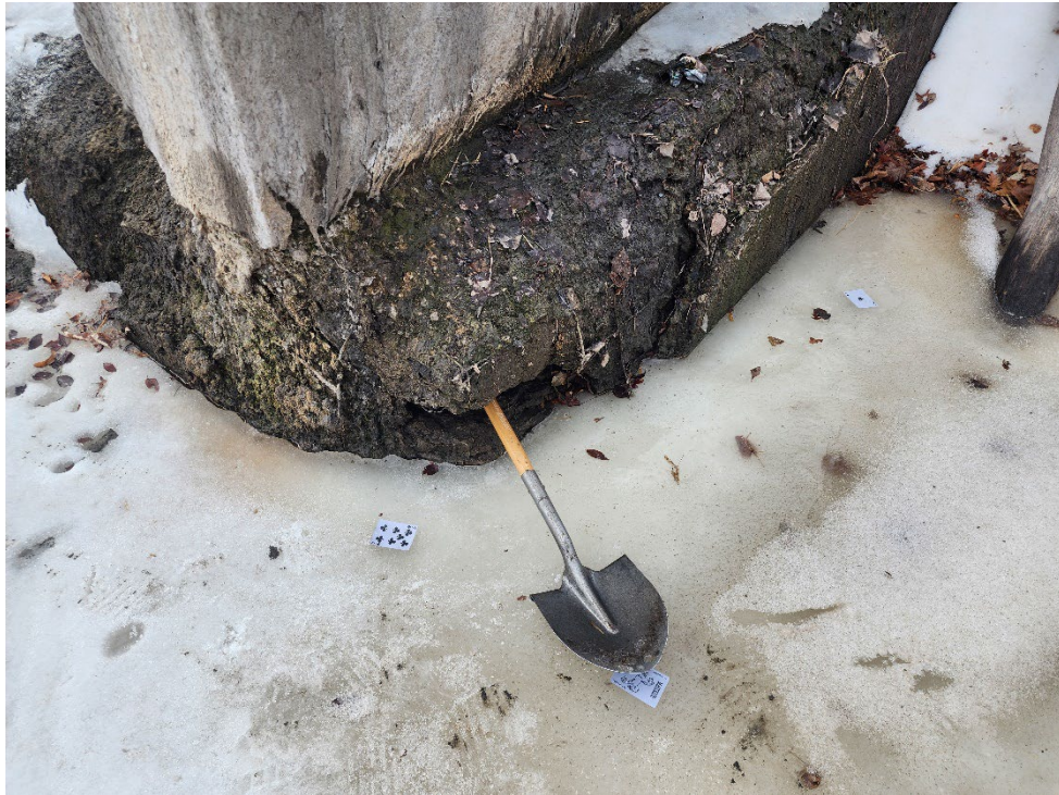
Photograph 25 Void in Base Slab of Dividing Wall Between Right Stop Log Section and Left Overflow Section
