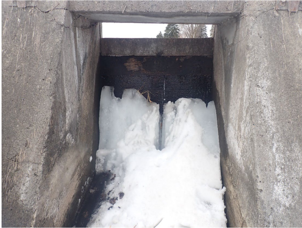
Photograph 18 Leakage Observed through Stop Logs
